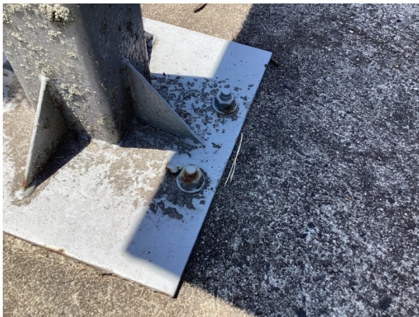
Mailbox station rusted fasteners
