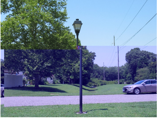
Light pole and fixture
